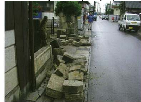
Photograph of collapsed stone masonry and concrete block walls following Northern Miyagi earthquake
