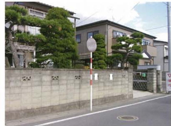
Cracked concrete block walls
